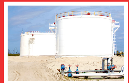
Remote Tank Monitoring
